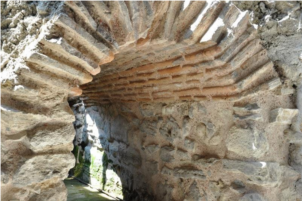
Underground passageways to the Hippodrome uncovered 2012-2014 when excavating behind the Turkish and Islamic Museum
